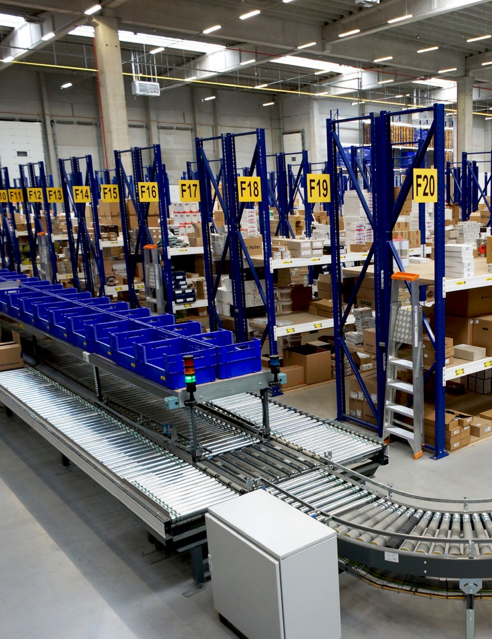
Automated order picking system for boxes and plastic crates for Satens Metaalwaren, Belgium
